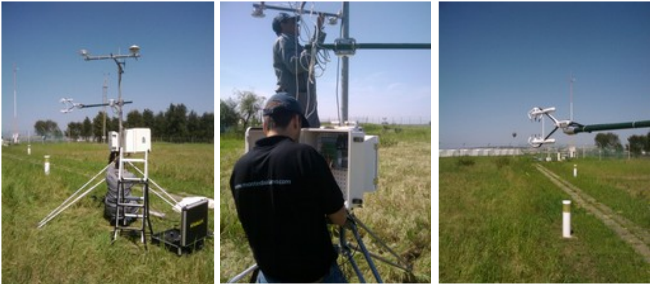
Figure 2.16 Installation of the IRGASON system in the Évora Regional Center of Meteorology
