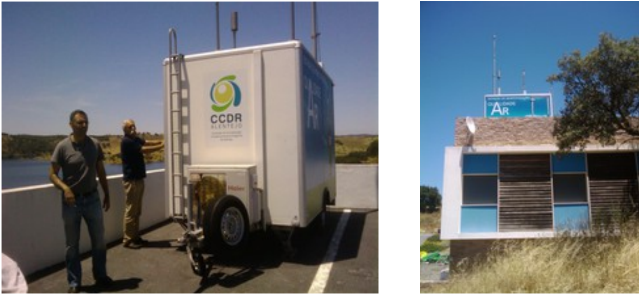
Figure 3.4 Installation of the air quality mobile unit in the boat park of the Amieira Marina. June 3, 2014.
