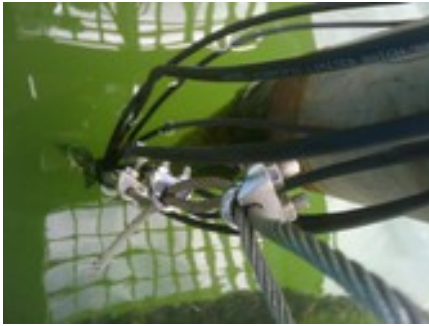
Figure 3.10: cables in which the water temperature sensors are attached
