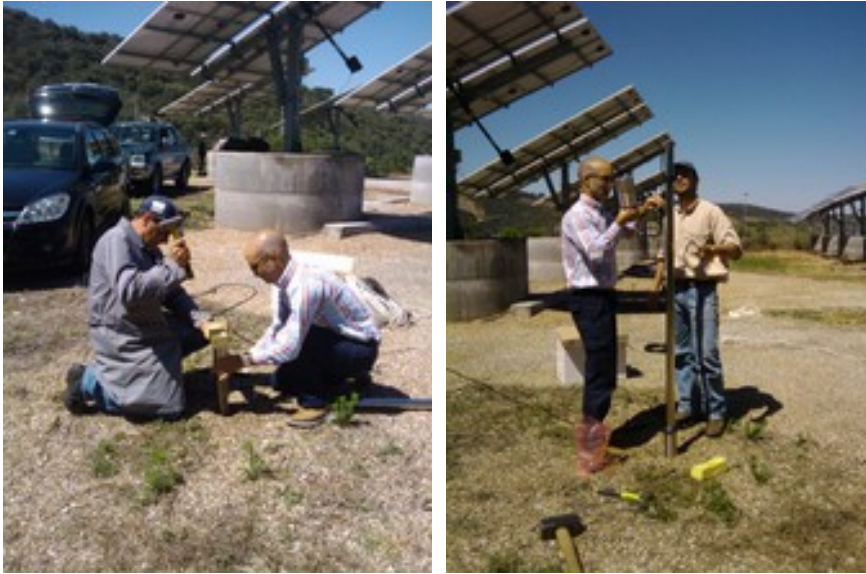
Figure 3.2 Instalation of an Electrostatic Fieldmeter at Solar Park experimental site
